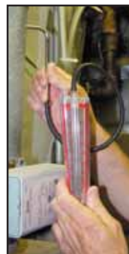
Furnace draft (left)
